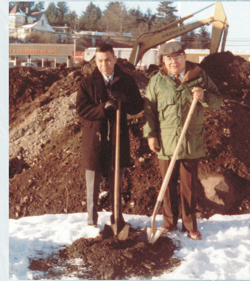
Director Gil Truitt and chairman Nelson Frank during the groundbreaking ceremony for the Shee Atiká Lodge.
